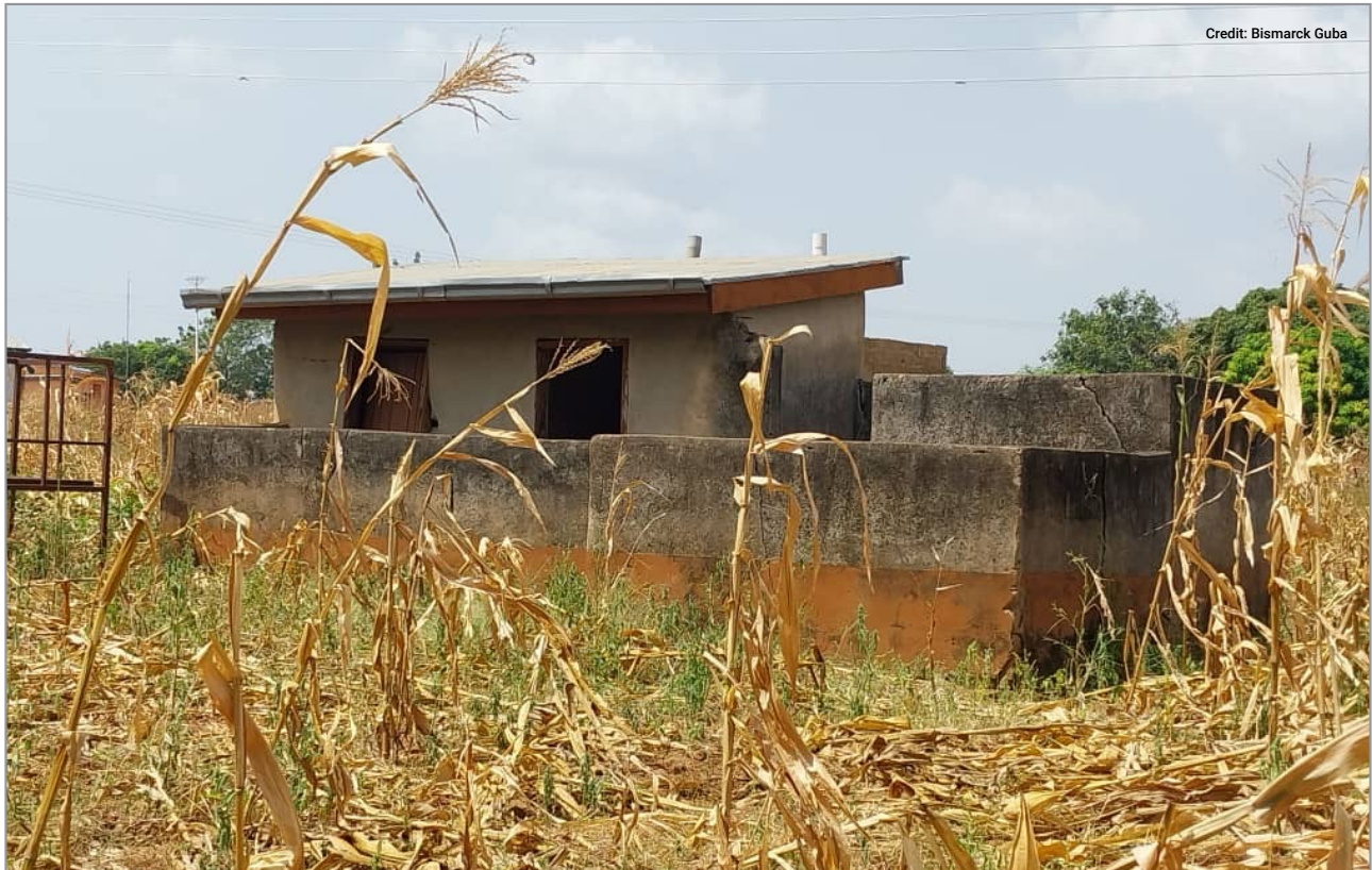
Photo 5.3. An abandoned public toilet in Bulinga, Bawku West, Upper East Region
